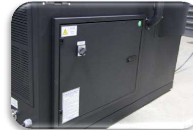
Concealed electrical panel
