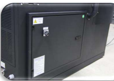
Concealed Electrical Panel
