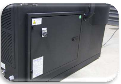
Concealed Electrical Panel
