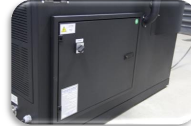
Concealed electrical panel
