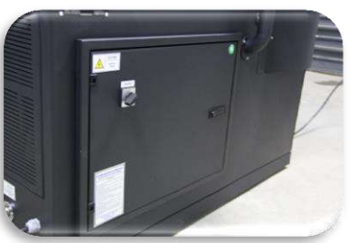
Concealed Electrical Panel
