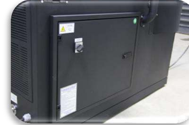
Concealed electrical panel
