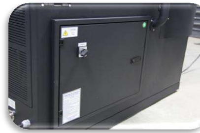
Concealed Electrical Panel
