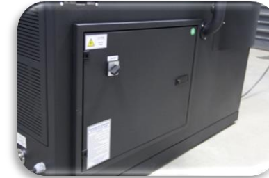
Concealed electrical panel
